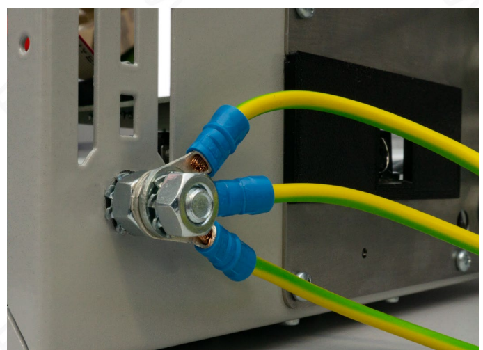
Fig. 24: Earth screw connection with attached cables.
