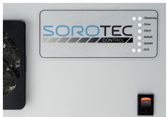
Fig. 17: The sticker seals unused holes
