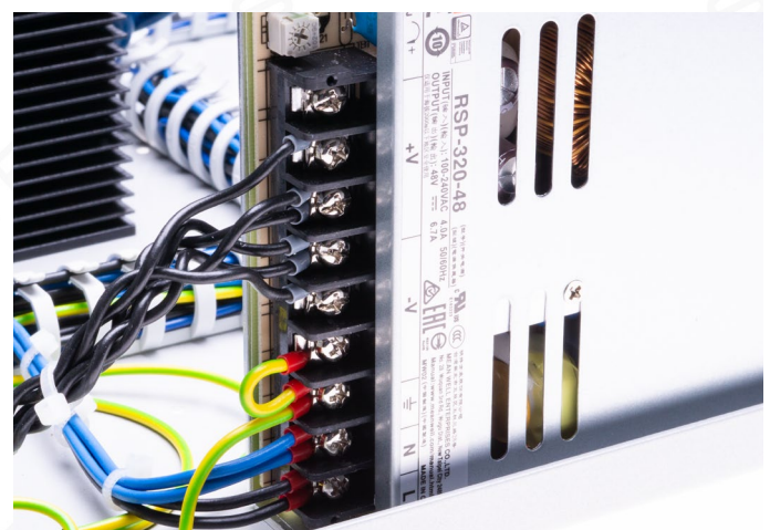
Fig. 15: The terminal block on the power supply
