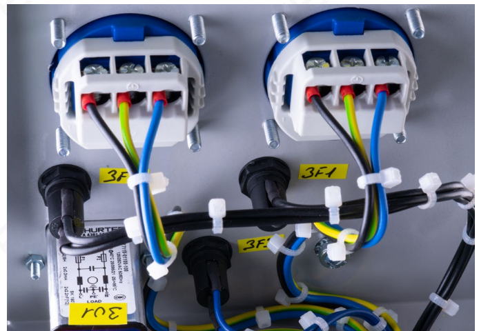
Fig. 17: The sockets for cooling and milling spindle
