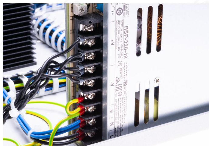
Fig. 18: The terminal block on the power supply
