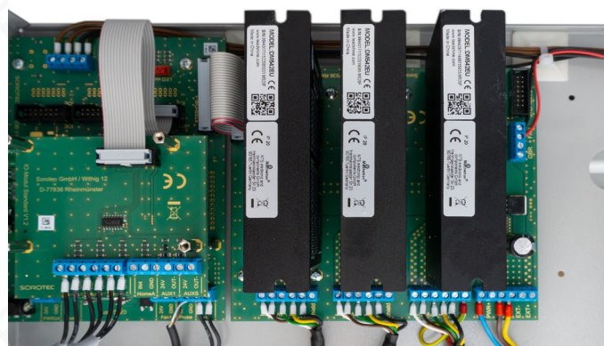
Fig. 27: Plugged-in power stages
