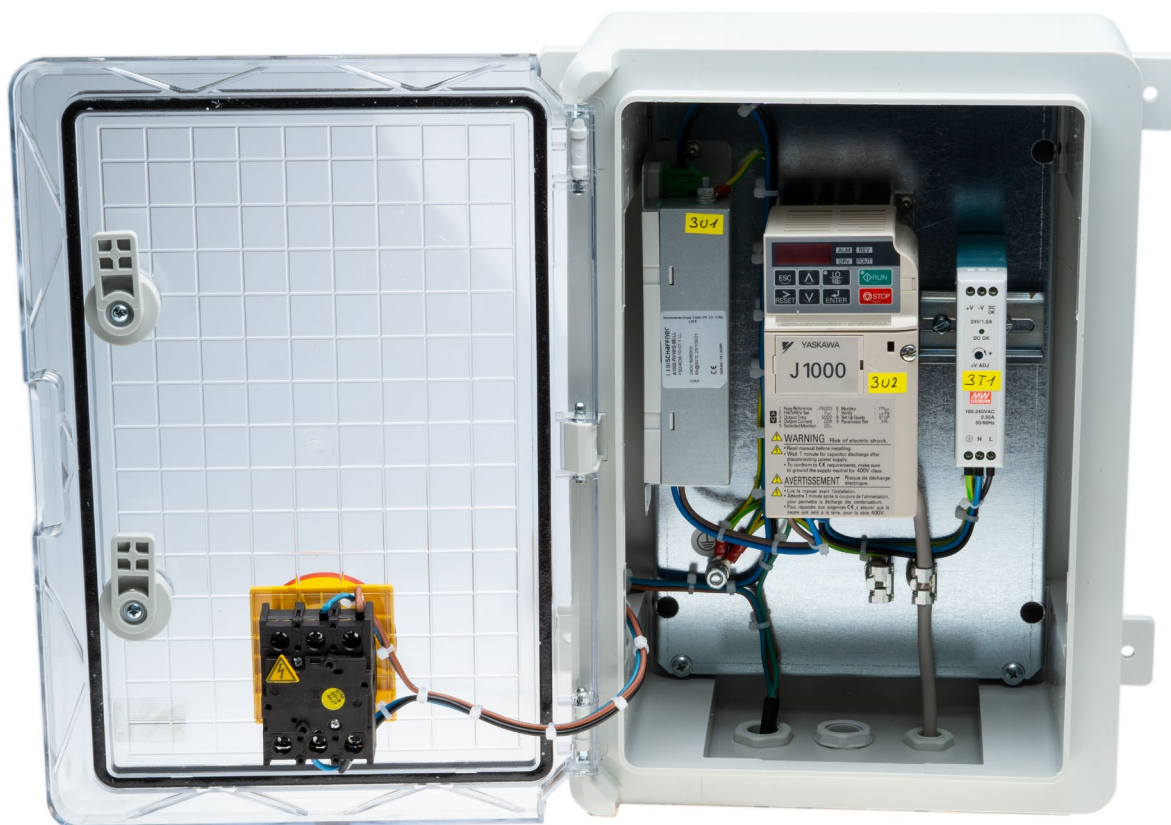
Figure 14: The fully wired control cabinet
